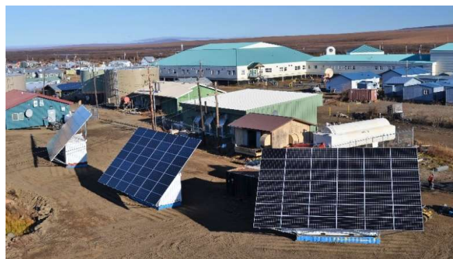
BoxPower’s SolarContainers powering a community in Buckland, Alaska
